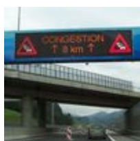
Variable message signs VMS LED
